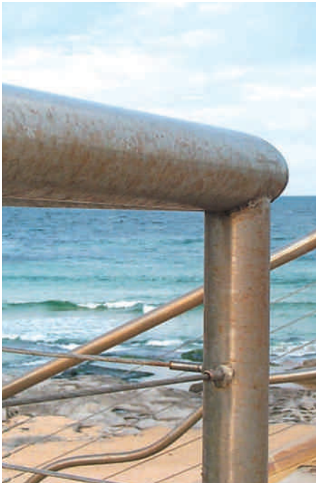
Tea staining of stainless steel in a coastal environment shortly after installation.
